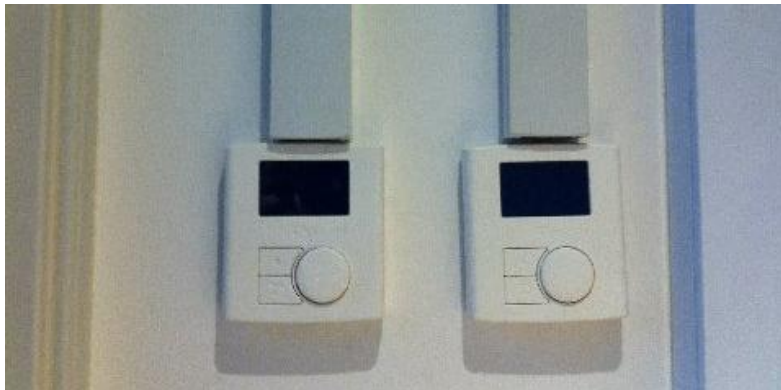
Mechanical Ventilation Heat Recovery System Controls
