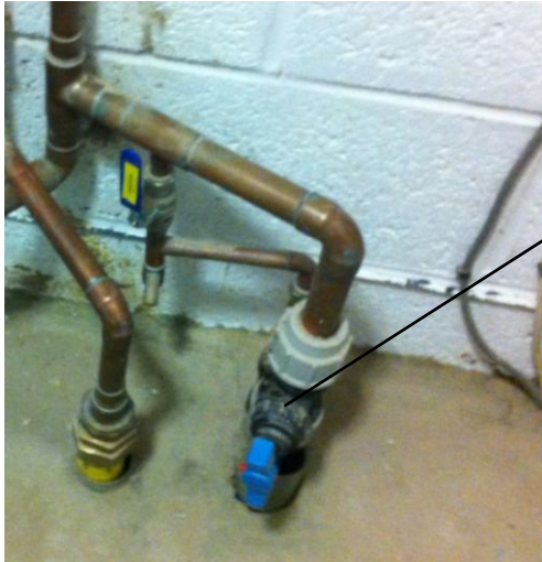
Incoming Mains Water Shut-Off Valve in Garage
