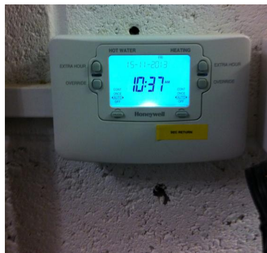
Heating and Hot Water Programmer
