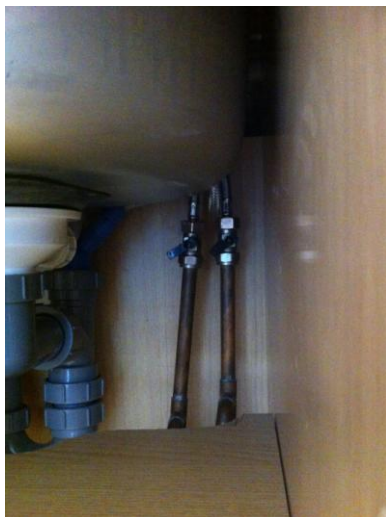
Shut-Off Valves under Each Sink
