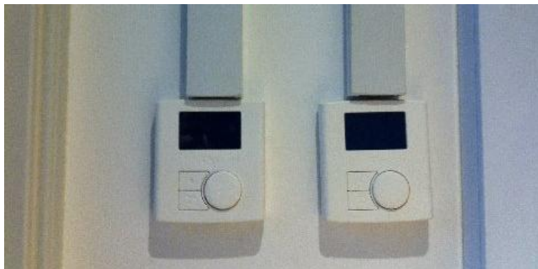
Mechanical Ventilation Heat Recovery System Controls
