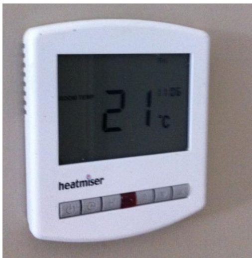
Underfloor Heating Controller
